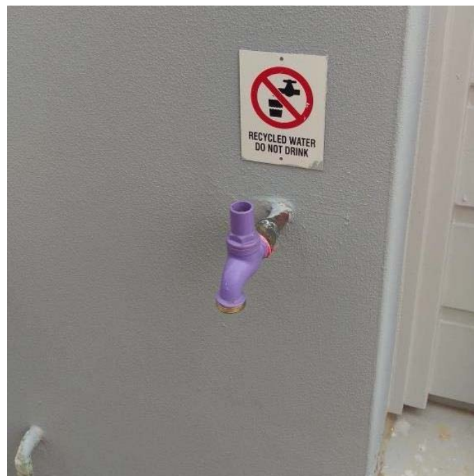
Figure D.3.4 Recycled water tap within a customer's property – lilac coloured tap with key (handle) removed and recycled water signage in place.
