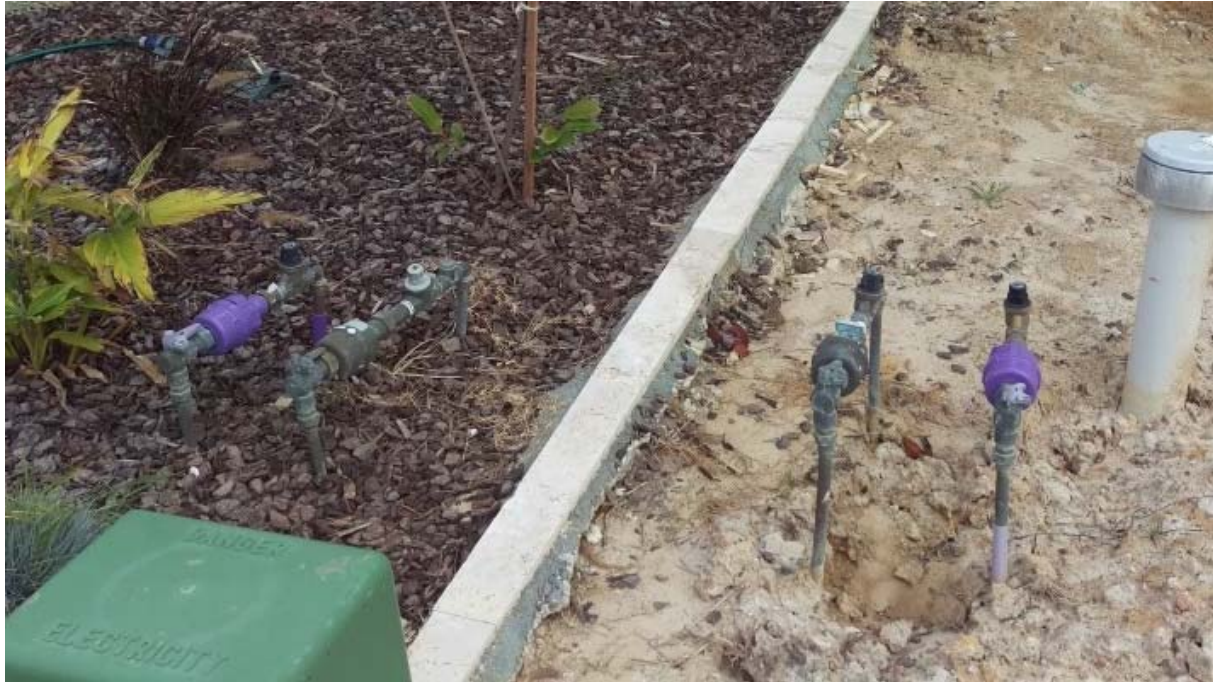
Figure D.3.3 Property connection installations with lilac sleeved risers and meter on recycled water connections.
