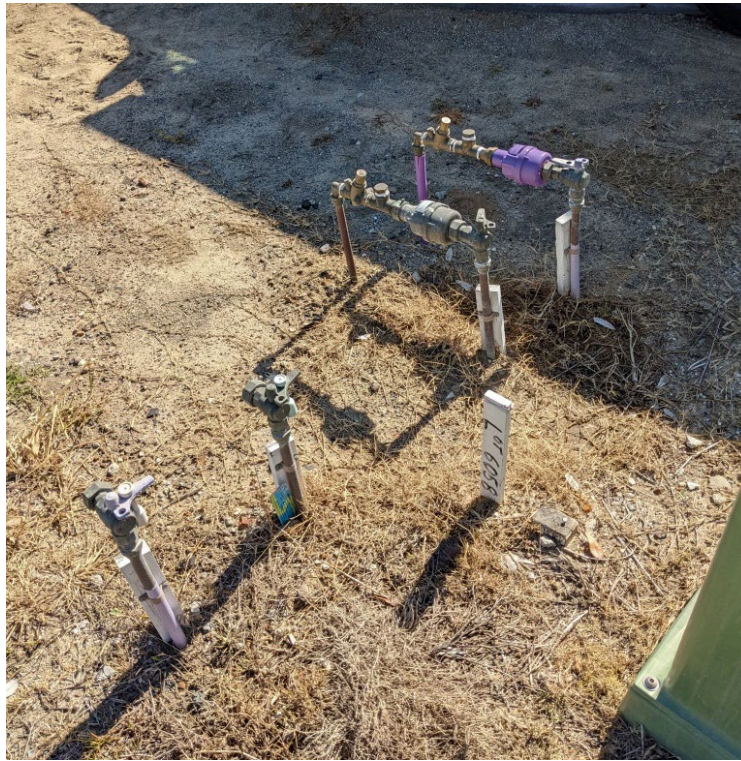
Figure D.1.1 Property connection installations with lilac sleeved risers and meter on recycled water connections. Note that valves are sealed and tagged to prevent use until authorised by Catherine Hill Bay Water.
